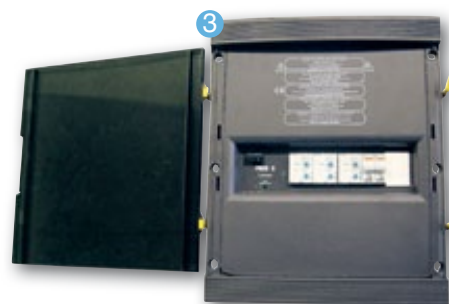
RED-3: Balance tank regulation control panel comprising 5 stainless steel sensors (ground, pump shut down, pump start up, solenoid valve open and close, overflow safety) and a 20/27 brass solenoid valve. Protected by a fuse.
